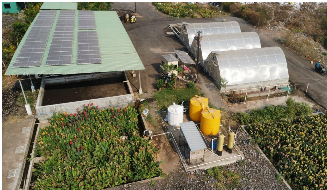
Figure 6: Covered sludge drying bed at Satara faecal sludge treatment plant, Maharashtra 2024 (Image source: CWAS)
